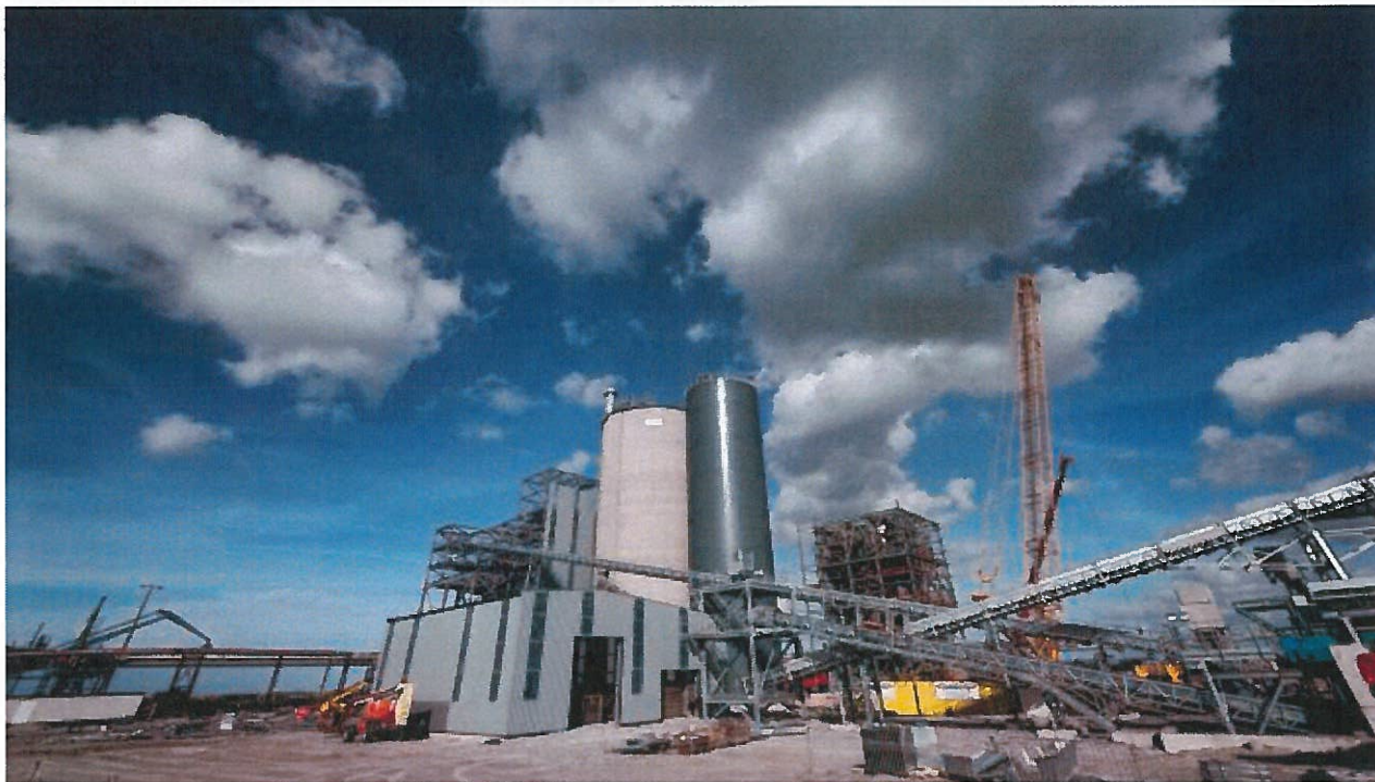
Ecocem's new plant under construction in Dunkirk. The election of the pro-business Emmanuel Macron as president has boosted business morale, according to company founder Donal O'Riain © Leo Novel/FT
